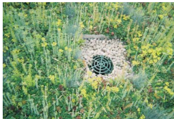
Roof drain within the new vegetated roof system
