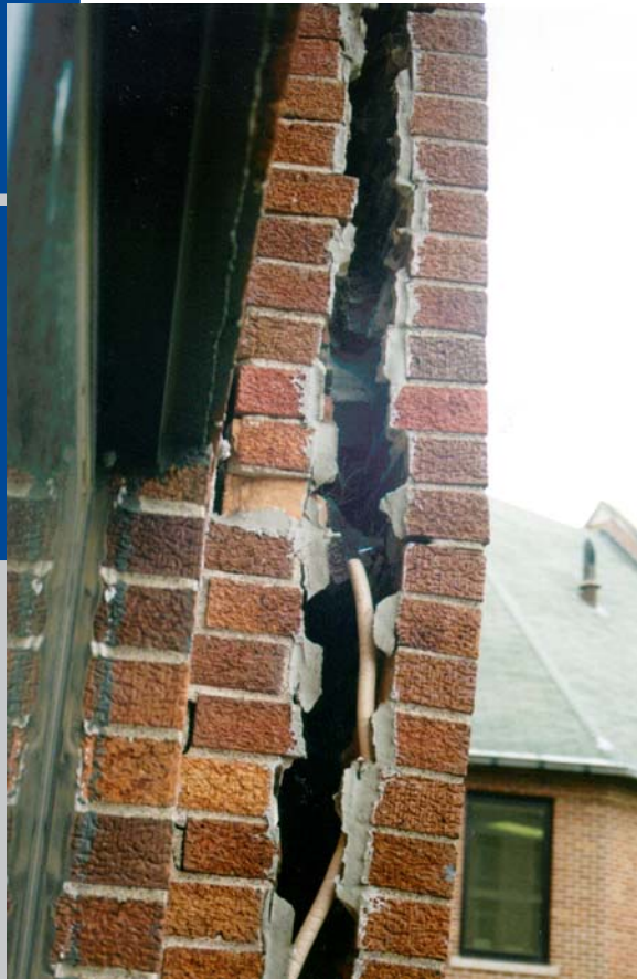
Exterior masonry brick is pulling away from interior wythe.
